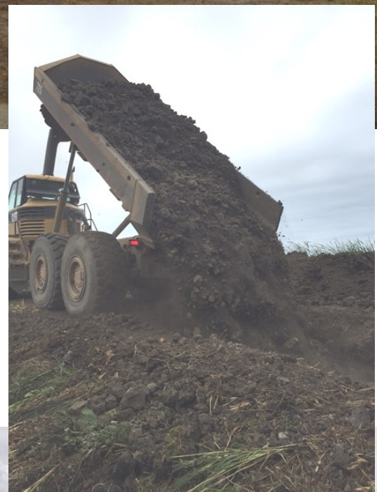
Above: Pair pond excavation to secure clay material for re-coring the dyke.
